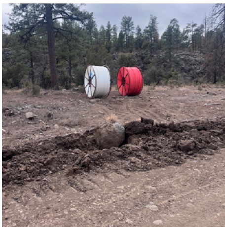
HIGH SPEED FIBER OPTIC CABLE READY TO BE INSTALLED
