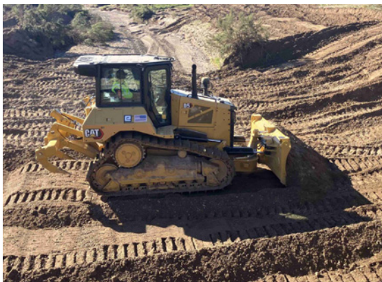
OCT 2025 FLOOD DAMAGE DOZER WORK TO REDUCE COMMUNITY RISKS
