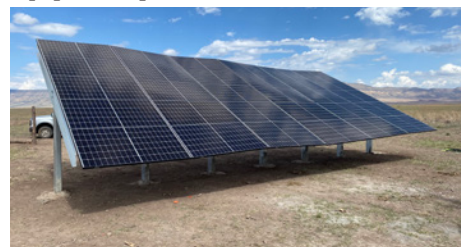
A SOLAR ARRAY POWERS A NEW WELL AT R-100
