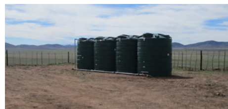
FULL WATER TANKS READY FOR USE
