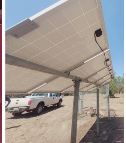
THE NEW STOCKWATERING FACILITIES WILL USE SOLAR-POWERED PANEL ARRAYS LIKE THIS ONE LOCATED IN BLOWOUT CREEK.
